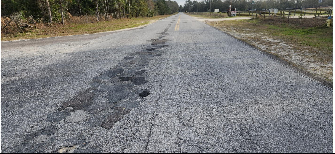
3. Hundreds of potholes with cold-patching, and severe alligator cracking.
