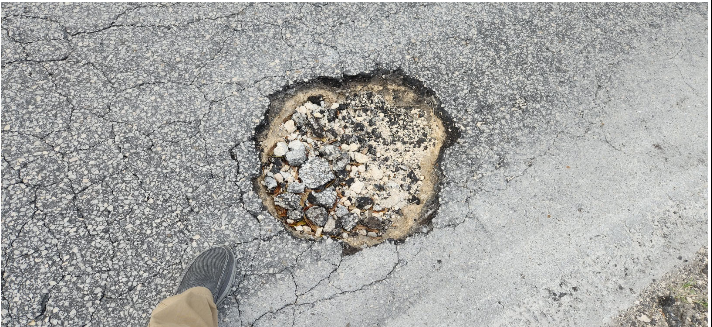
6. Large and deep potholes open up after every heavy rain.
