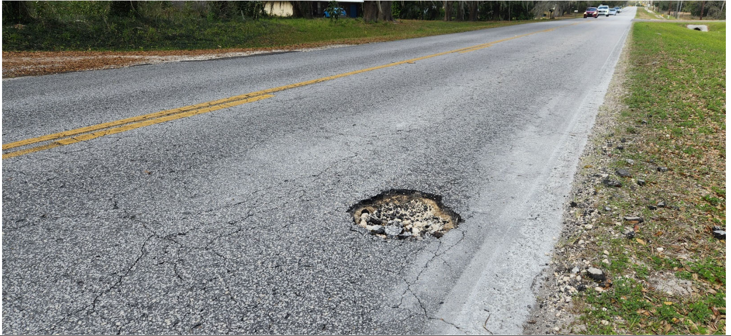
5. Large potholes in travel lanes force vehicles to swerve into on-coming travel lane or off the pavement, causing edge crumbling.
