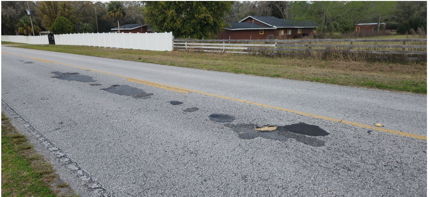
10. North end of SW 75 th looking towards Brytan. Note rutting & potholes.
